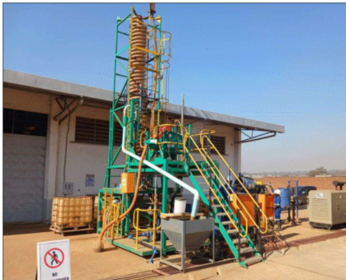
Figure 1: Installed Spiral plant at Sovereign's Lilongwe facility
